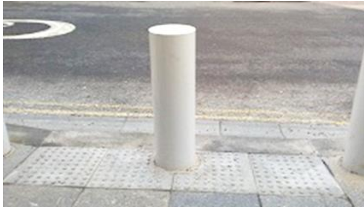
Bollard obstructing tactile paving and dropped kerb
