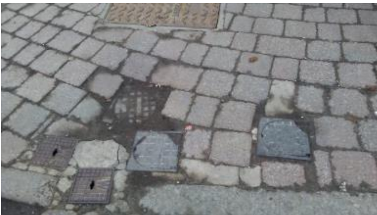
Poor footway at entrance to Fisher's Hotel car park
