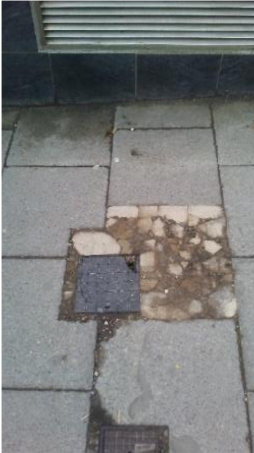
Poor footway outside Keepsakes
