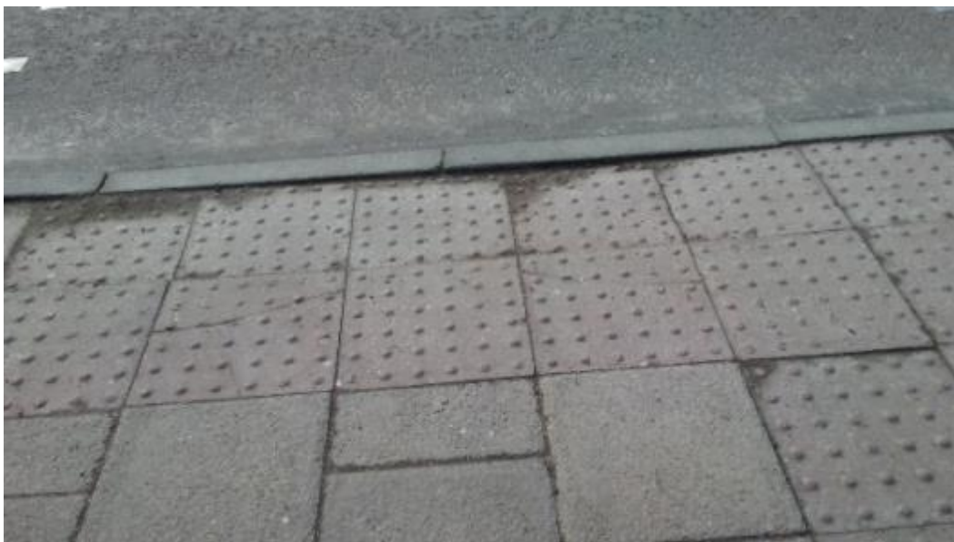
Poorly maintained dropped kerb
