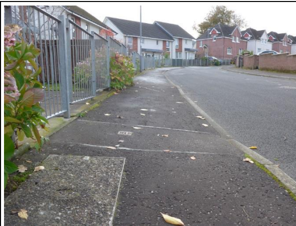
Footway crossover to private driveway (problematic crossfall/slope over whole footway width)
