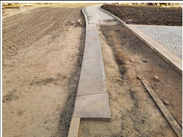
Dutch-style entrance kerbs (by Charcon) being added at a footway crossover (to a private driveway) in a new residential development, to create a level footway (photo © courtesy of Aberdeenshire Council)
