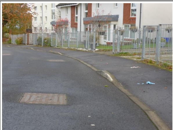
Footway crossovers along a longer stretch of footway (problematic crossfall/slope throughout)
